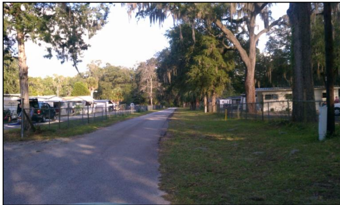
Photographed while looking East on NE 32nd St. at the intersection with NE 56th Ave. This stretch of pavement fails to include curbs, gutters, sidewalks, or any form of stormwater infrastructure. The pavement is crumbling on the edges.
