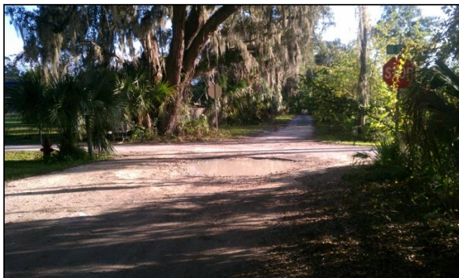
Photographed at the Intersection of NE 57nd Ave. and NE 32nd St. This is a dirt road in a residential area. As a result of the lack of pavement, severe ponding has occurred in the middle of the dirt road adjacent to the stop sign.
