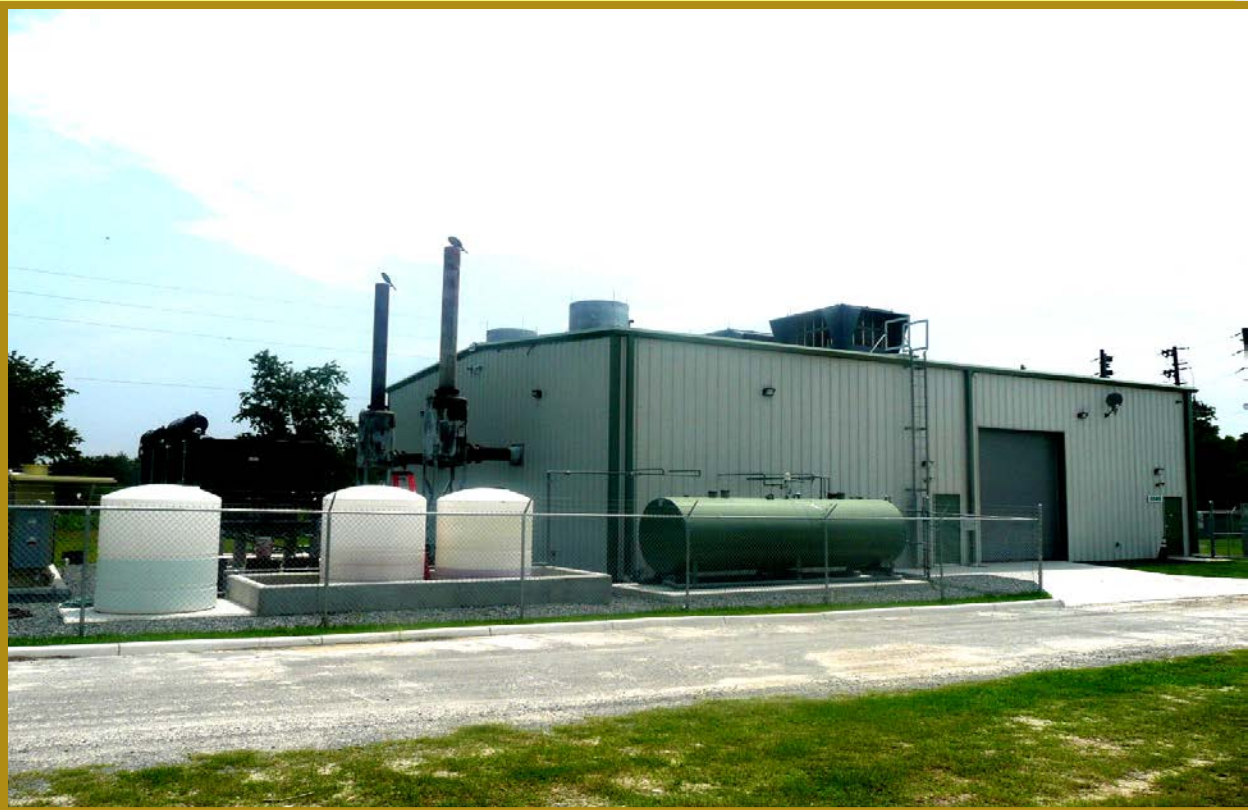
G2 Energy Plant
